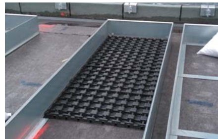
A build-up with Aquatec® AT 45 was used within the frames of the planting beds, and one with Floradrain® FD 40-E in the surrounding area.
