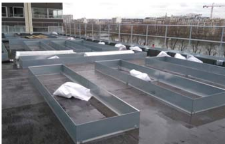
The metal frames with ca. 350 mm of height were positioned directly on the Protection Mat ISM 50, which covers the entire roof area.
